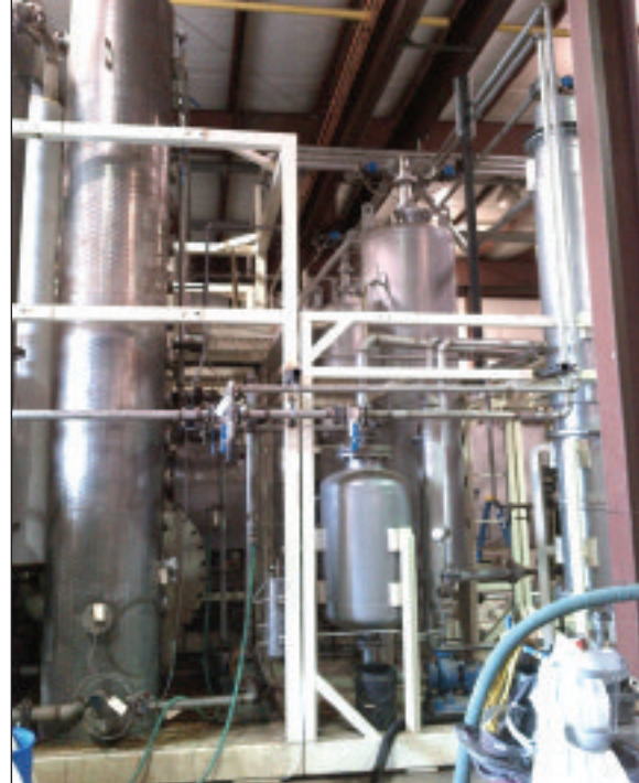
Green Biologics will install new distillation equipment for renewable n-butanol and acetone adjacent to Easy Energy's existing distillation unit.
